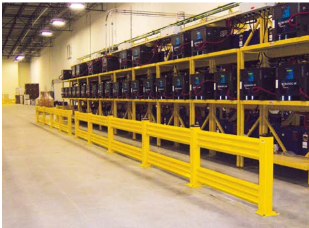
Guarding battery racks
