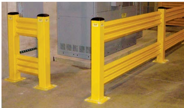
Guarding electrical panels
